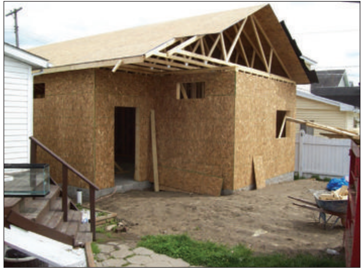
The amazing before and after photo of the exact same area at the GGGH as the foundation goes in, top, and then new structure!
